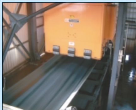
Eriez magnet installation in China
