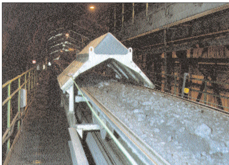
Figure 2. NGCQM installed on a run-of-mine conveyor belt.
